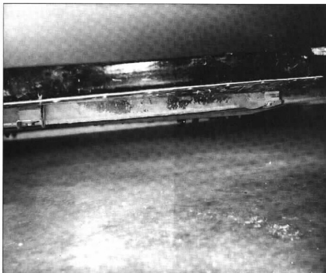
Above: The new hog trough installed. Note the frame bolts and shims.
