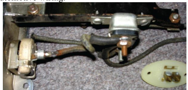
Left: Switch using bullet type connector Center: Breaker with studs using wire terminals with loops. Right: Pillar switch with screws. Wire terminals used will be loops.
